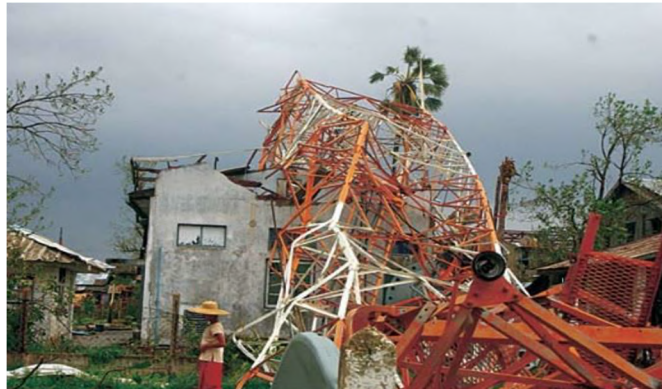
Fig. 2.20 : Damage of communication towers due to cyclonic wind
