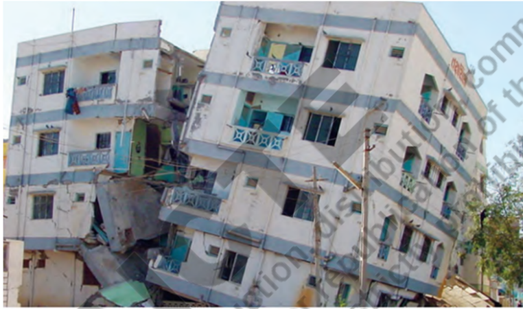
Fig.2.1: Building damaged due to Gujarat 2001 earthquake
