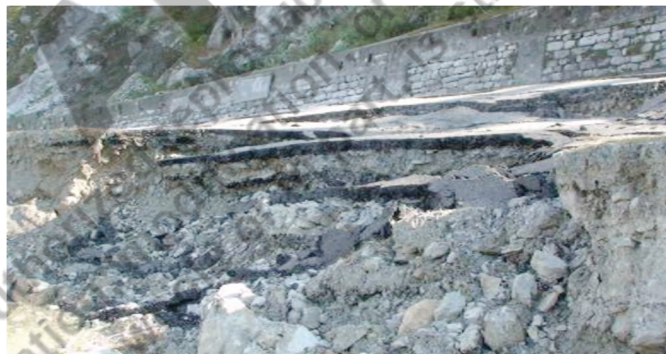
Fig. 2.38: Example of lateral spreading
