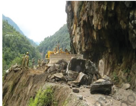
Fig. 2.30: Example of Failure in Fall
